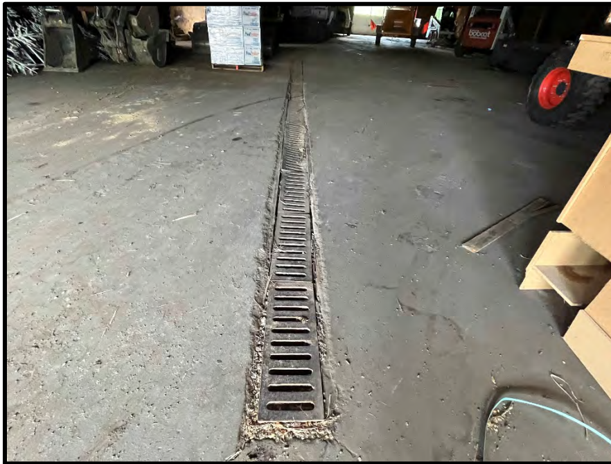
VIEW OF TRENCH DRAIN LOCATED IN THE WESTERN PORTION OF SUBJECT BUILDING
