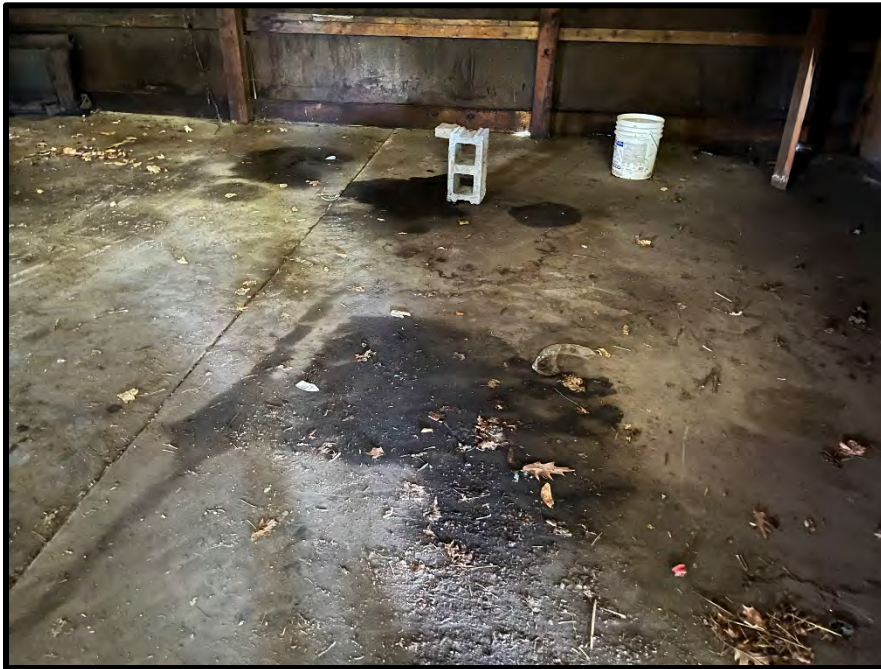
VIEW OF OIL STAINING IN THE SOUTHERN CENTRAL PORTION OF THE SUBJECT BUILDING
