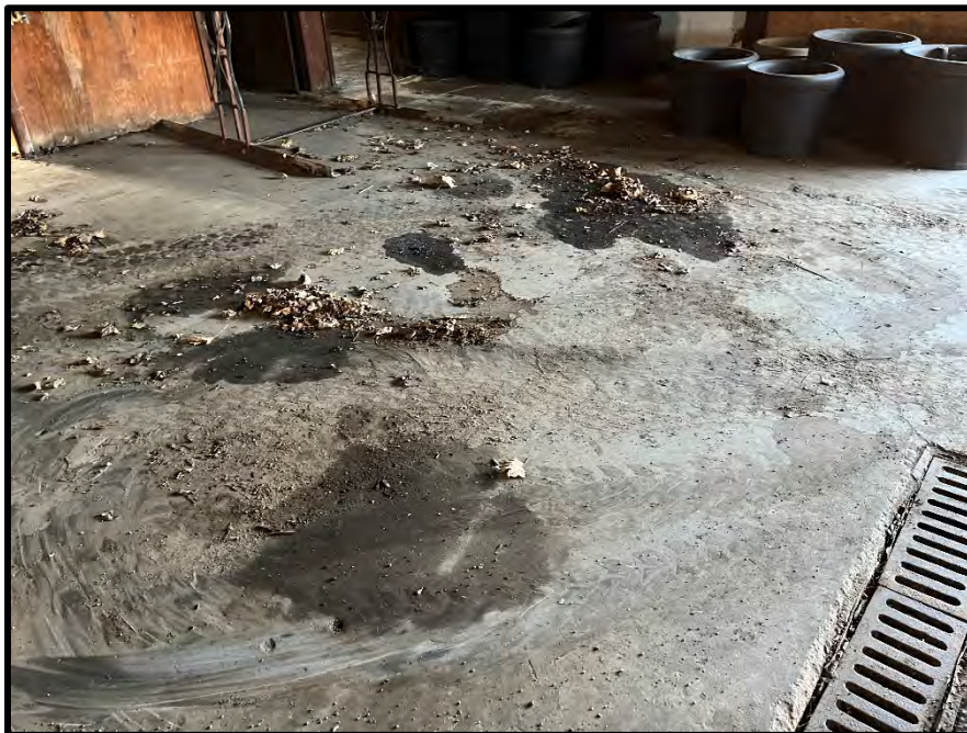
VIEW OF OIL STAINING LOCATED IN WESTERN CENTRAL PORTION OF SUBJECT BUILDING
