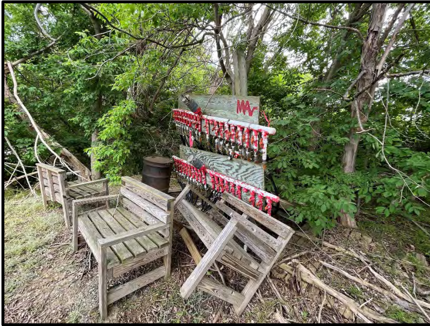
VIEW OF REMEDIAL SYSTEM LOCATED ON THE SOUTHEASTERN CORNER OF THE SUBJECT PROPERTY
